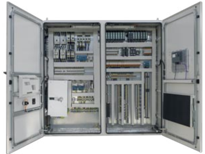
Switchgear & Control Cubicle
